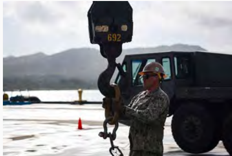
Crane lift: Seabees, assigned to Naval Mobile Construction Battalion (NMCB) 133, conduct a crane lift on a pier in Santa Rita, Guam, April 16, 2025.
