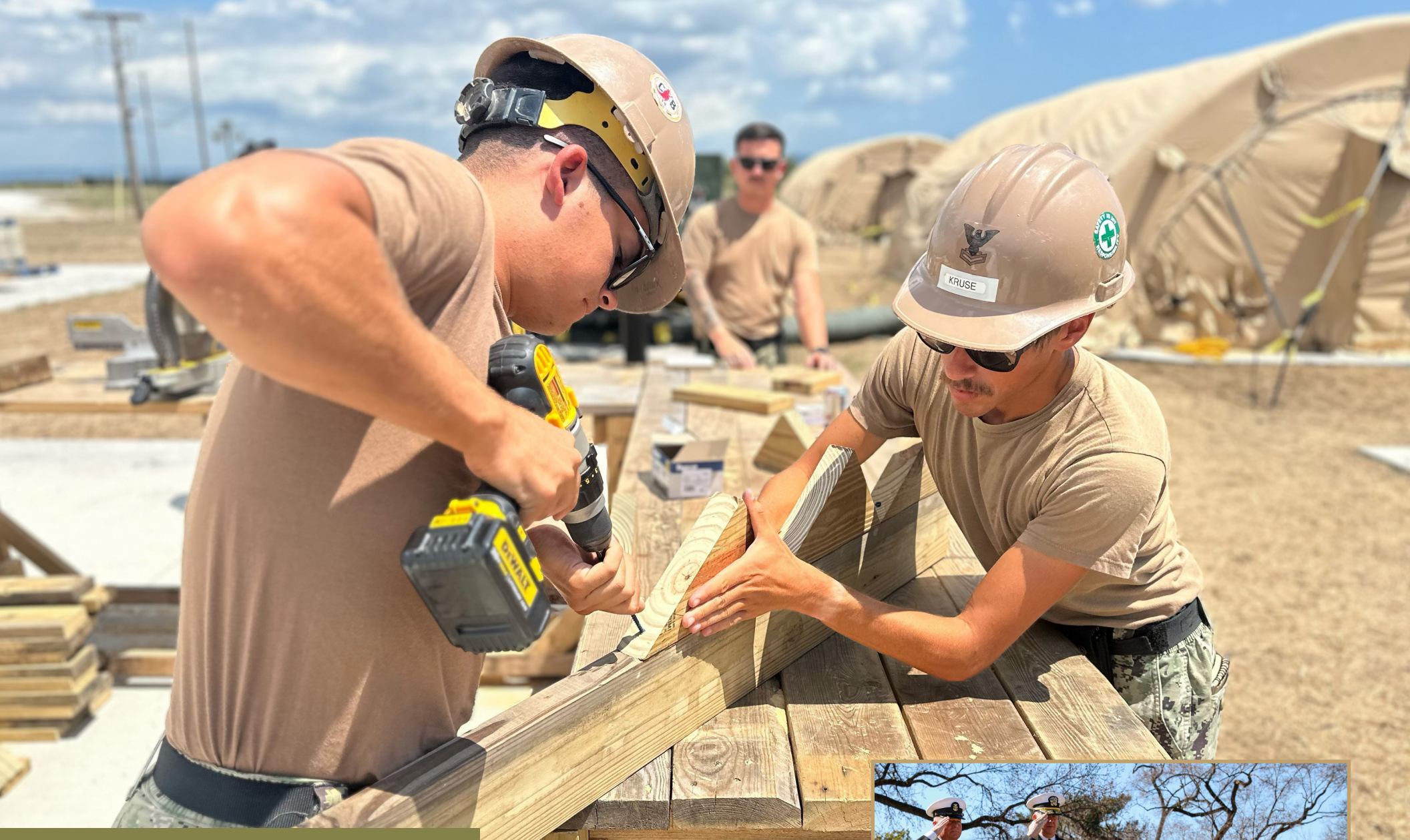
GUANTANAMO BAY CUBA (MAR. 12, 2025) - Seabees assigned to NMCB 133 build stairs for the Department of Homeland Security migrant operations center at JTF-SC supporting illegal aliens holding operations led by the Department of Homeland Security at Naval Station Guantanamo Bay, Cuba. (U.S. Army photo by Sgt. 1st Class ShaTyra Cox) (Sgt. 1st Class ShaTyra Reed-Cox)
